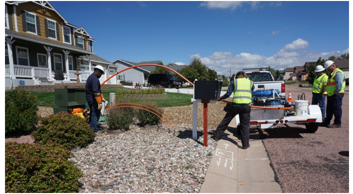
Microduct technology and contractor collaboration have enhanced the efficiency and progress of MVEA's fiber project.
