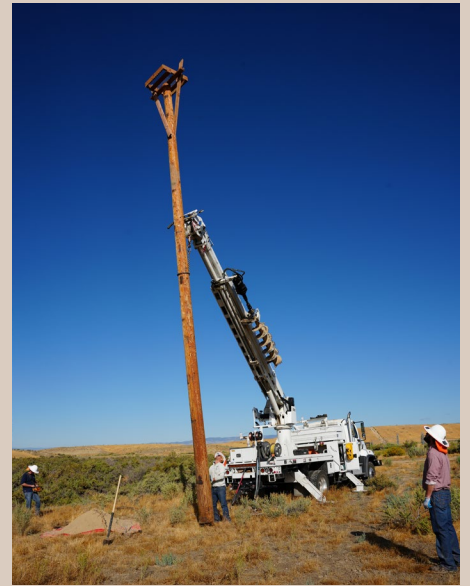
▲ A Grand Valley Power linecrew installs an osprey nesting platform in Highline Lake State Park.
