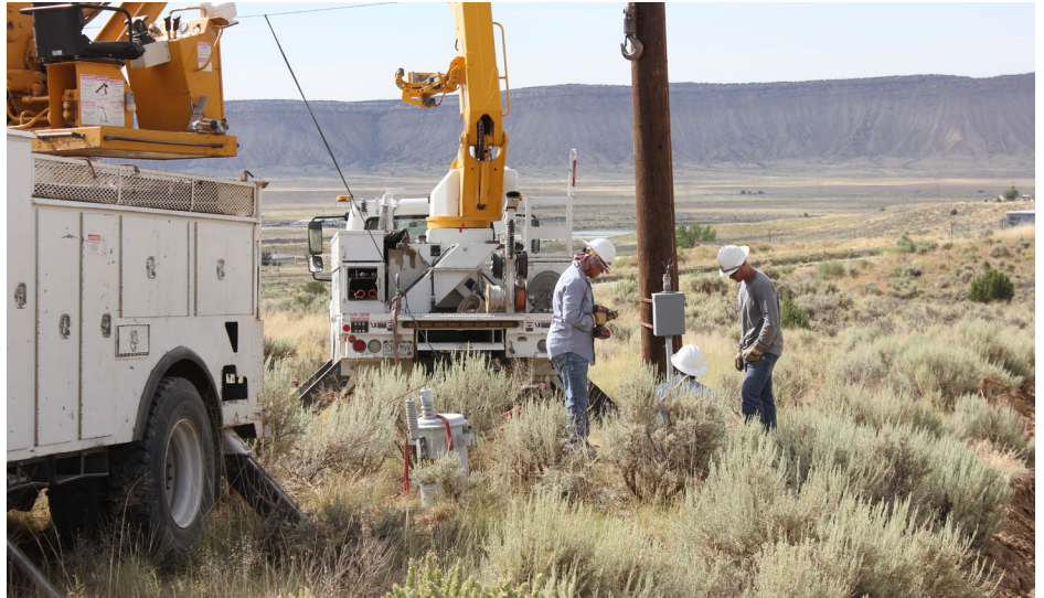
EEA linemen Shad Bellmire, Matt Ruggles, and Justin Purkat replace a pole-mounted service as part of the Towaoc alternate feed project.
