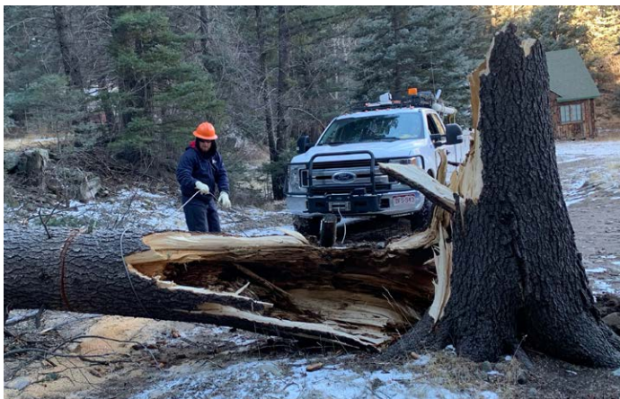
▲ SIEA lineworker works safely to clear a massive fallen tree from downed power lines using a truck winch.
