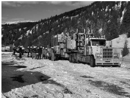
▲ GCEA linemen work with the Tri-State crew to assemble a mobile substation to help with the outage in Lake City.
