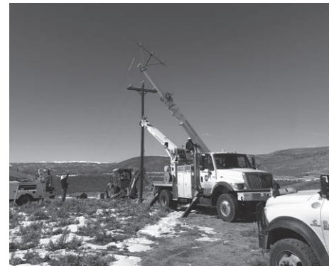
▲ GCEA linemen work on a pole to restore power during an outage.
