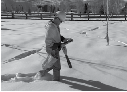
▲ GCEA Lineman Ty Percival performs a line locate for underground power lines.
