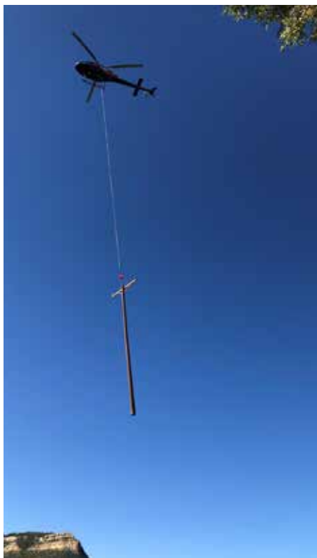
A new power pole is airlifted to the job site. Photo courtesy of Orly Lucero.
