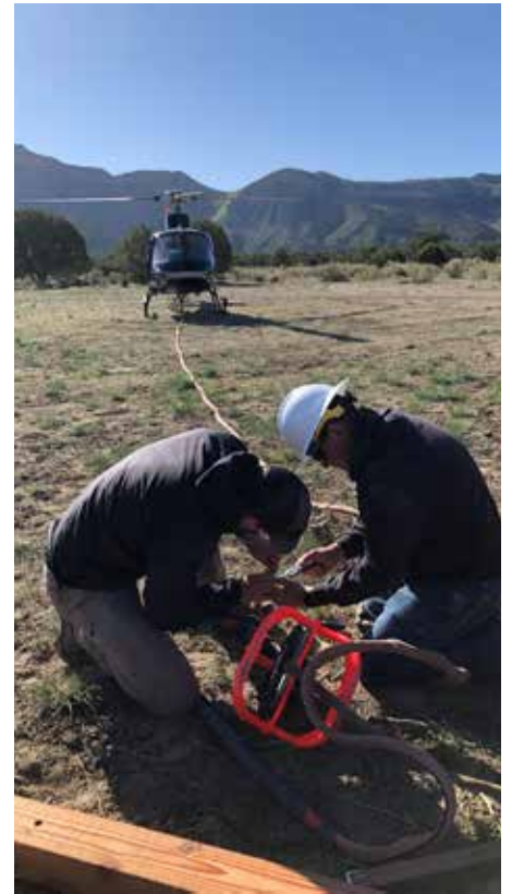
EEA's Brad Dennison (right) assists the helicopter ground crew prepare the harness used to transport poles to the job site. Photo courtesy of Orly Lucero.
