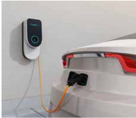
▲ A Level 2 electric vehicle charger can overload EEA's equipment serving your home.
