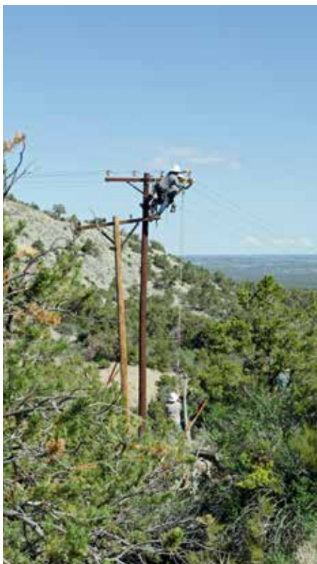
Nick Podrazik and Justin Purkat secure insulators on de-energized line with assistance from Jake Thurman and Tyler Berry. Photo courtesy of Ace Astor.
