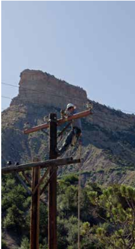
Chase Suckla attaches conductors to a new pole prior to re-energizing the line. Photo courtesy of Ace Astor.
