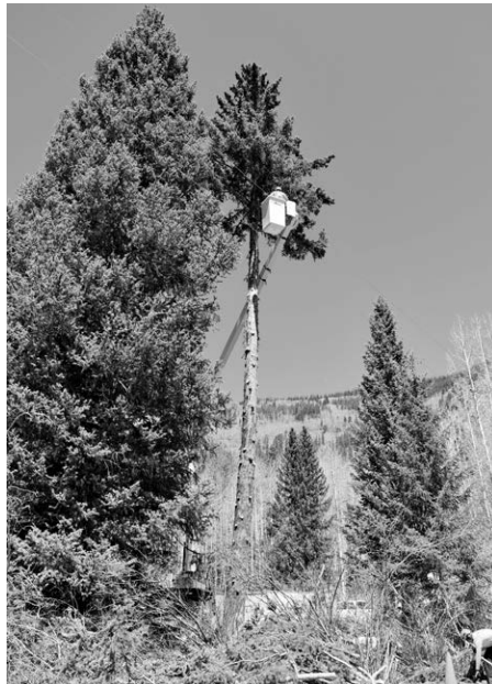
▲ Skilled, time-consuming work and an investment in specialized equipment is necessary to safely clear lines of vegetation around power lines.
