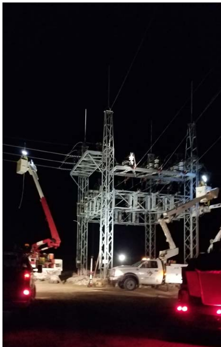
2019 Keystone Substation upgrade. YVEA crews worked through the night to complete the project.
