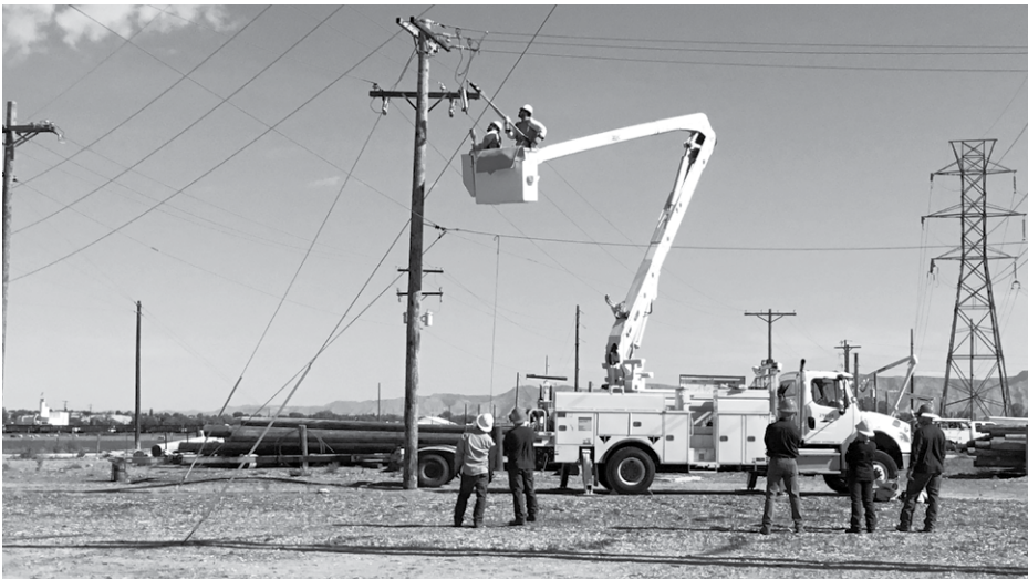
Seth Baker and Carson Ebke work from a bucket truck at Hotline School. Photo by Jeff Poe.
